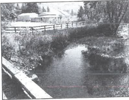
Eroding creek bank by bridge. View to NE.
